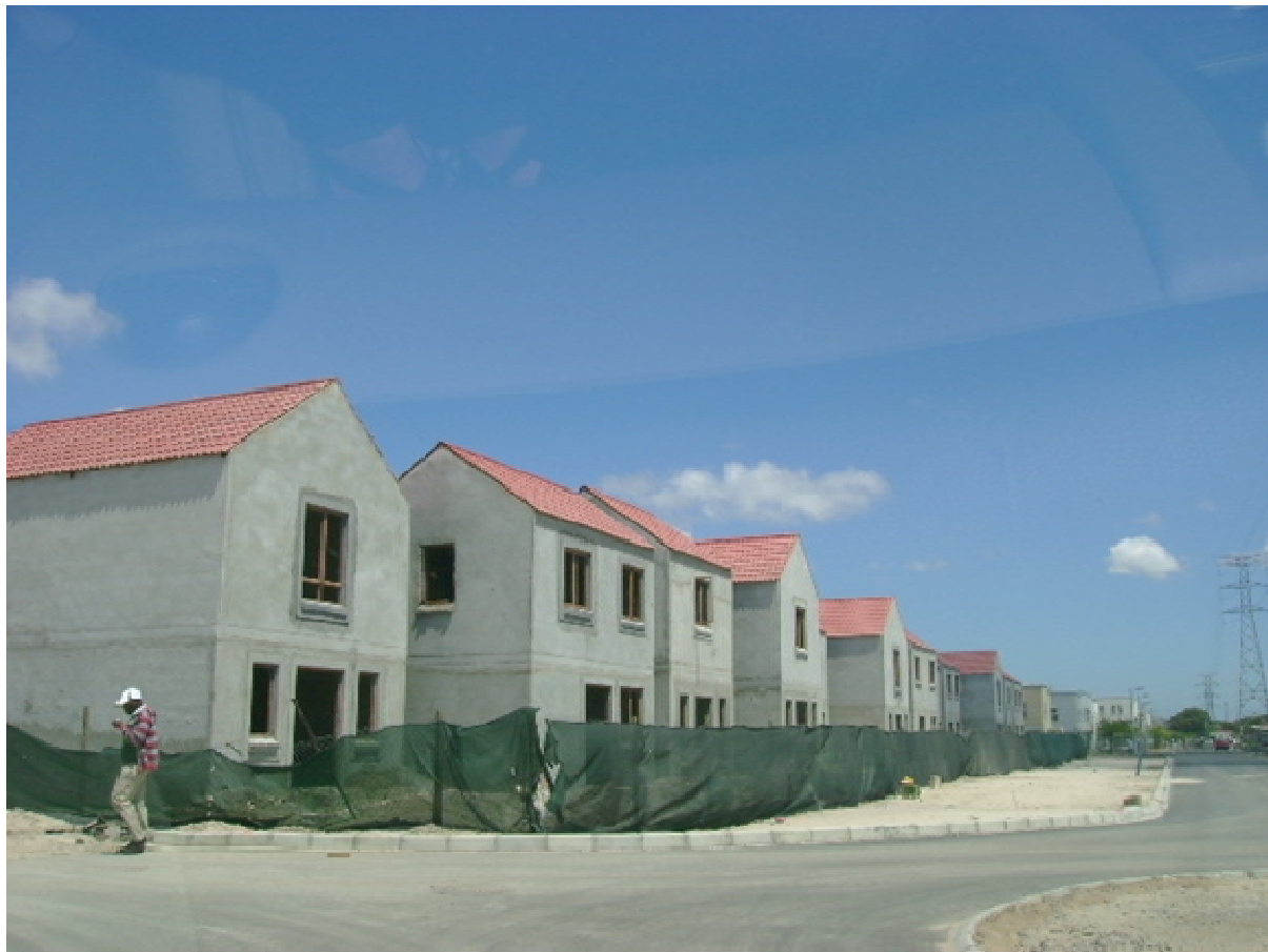
Credit-linked bond houses under construction as part of Phase 2 of the N2 Gateway project
